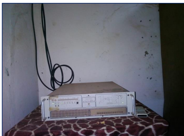
Transmitter room, Brikama Ba CRS
