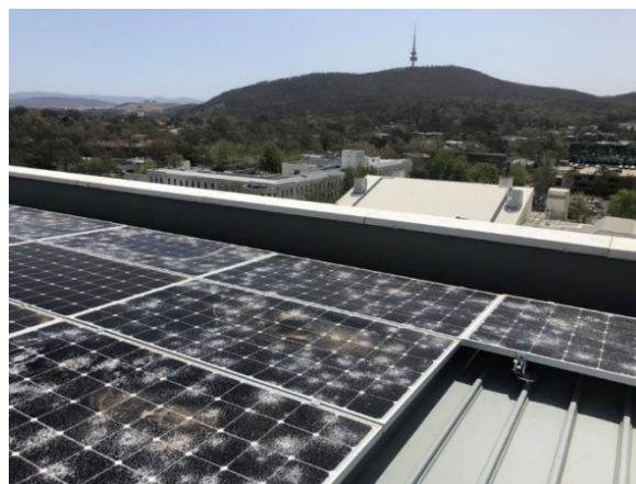
Figure 11: Hail damaged solar panels in Canberra 40
