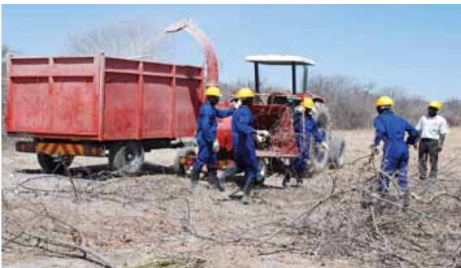
Clearing land for grazing while simultaneously supplying Namibia with clean, renewable electricity.
